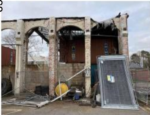
Central brick arcading with missing roof
